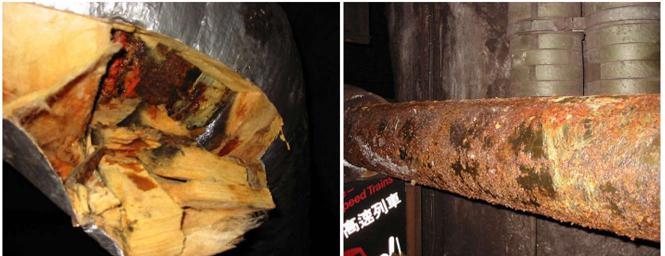
Figure 2: Examples of UIC effects on metal pipe work insulated with traditional mineral wool/metal cladding systems after only a few years of service.
