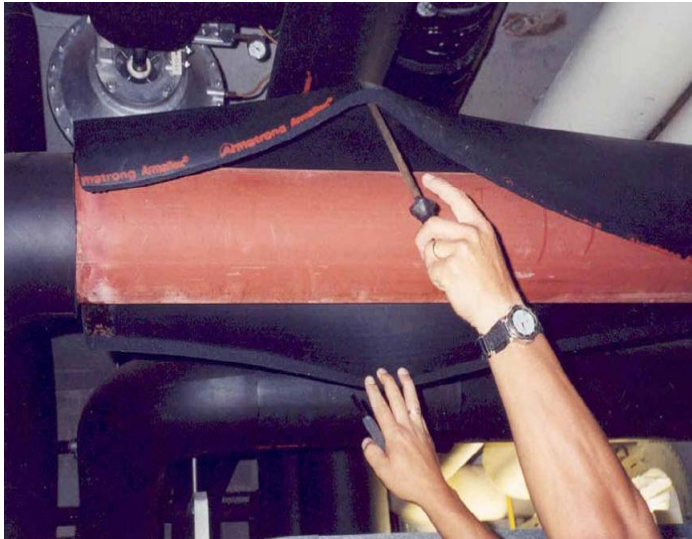
Figure 4: Example of cold water pipeline which has been insulated with closed cell insulation (Armaflex) for more than 20 years.
